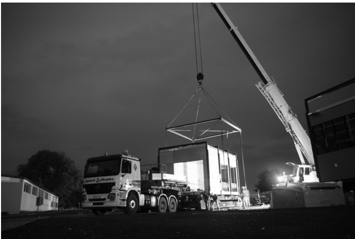
Figure 2. The two house modules prepared for the initial lift. The spanner beams had failed the previous evening. Photo by David To, Arganda del Rey, Spain, 2010.
