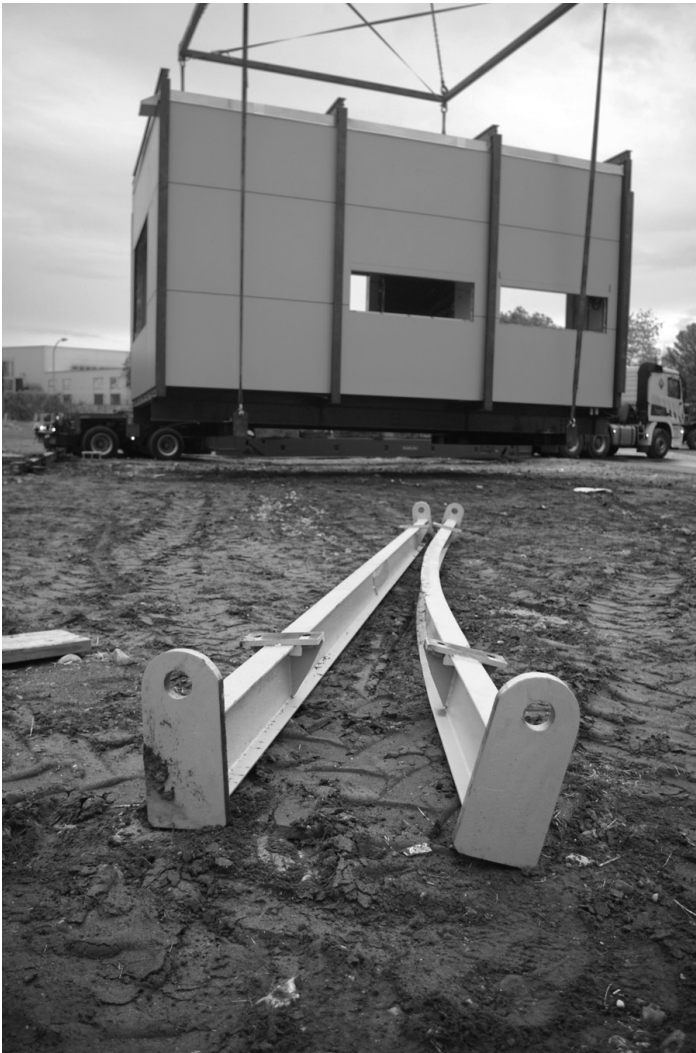
Figure 4. Failed spanner beams with the RE:FOCUS house in the background. Photo by David To Arganda del Rey, Spain. 2010
